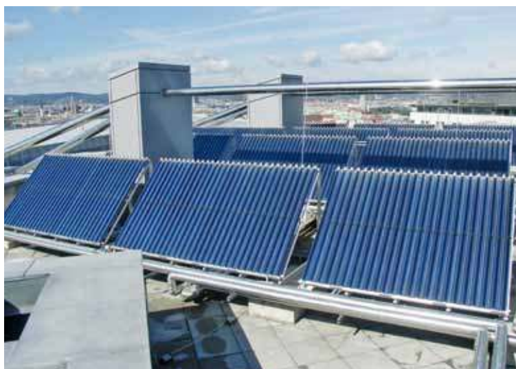
Solar collectors on the roof of the Vienna head office
